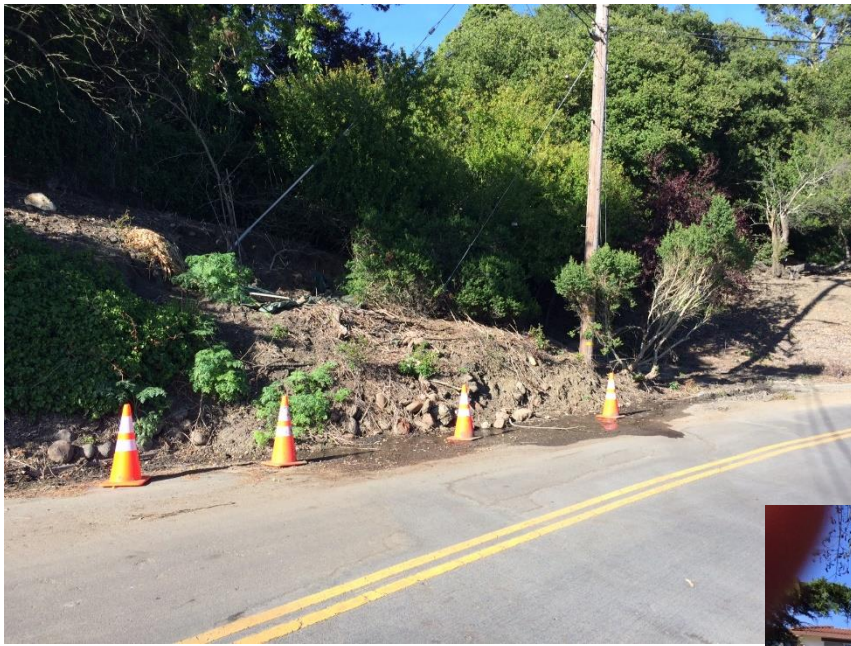
Small mudslide and spring on Havens Place
